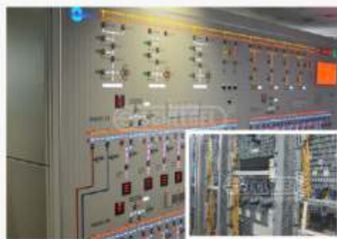
Control Monitoring Panel / Mosaic Mimic Panel
